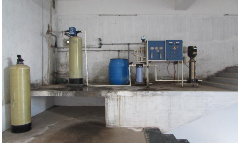
RO Water Plant
